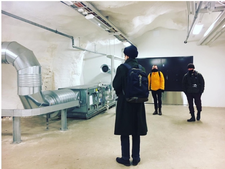
The corridor of VTT. Timo Viialainen observing the ventilation system. Joonas Mäkelä as well as Teppo Vesikukka from the VTT administration are included in the image. © Fjolla Hoxha
