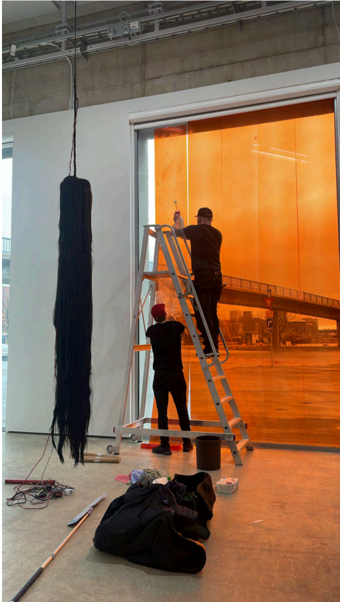
17.04.2024 Window installation company called Easytape installing the films. Photo by Soyoung Christina Chung
